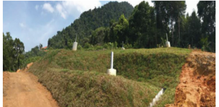
500kV OHL Bentong South-Lenggeng
