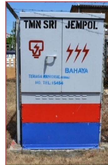
LV FEEDER PILLAR (415/240V)
