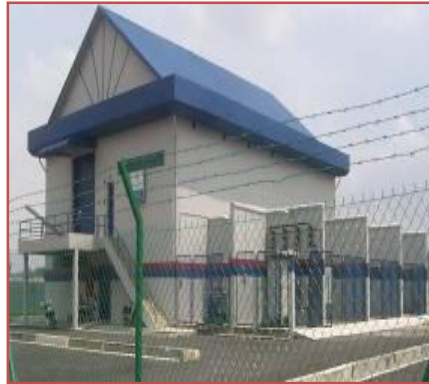
DISTRIBUTION MAIN INTAKE 33kV/22kV
