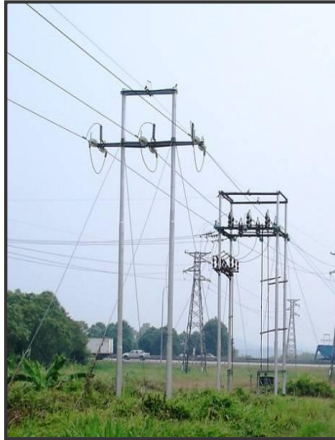
DISTRIBUTION TOWER 33kV/22kV/11kV
