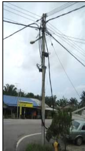
LV OVERHEAD LINES (415/240V)
