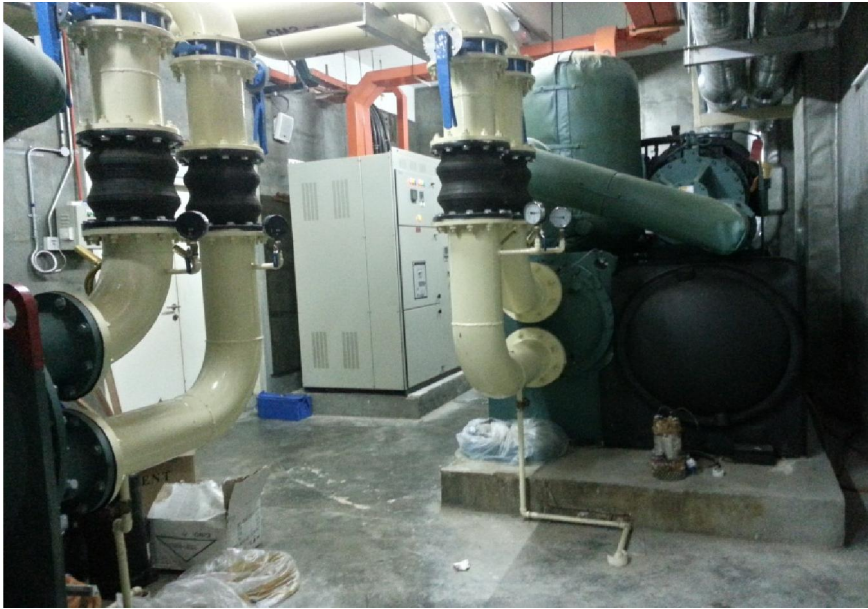
Chiller: 320RT x 2 unit
