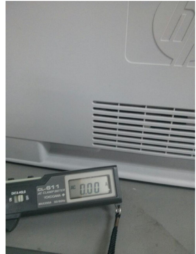
Power supply 13A: OFF
