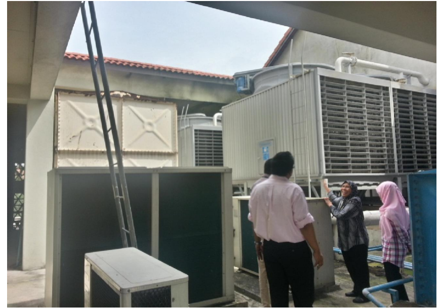
Cooling Tower: 2 unit
