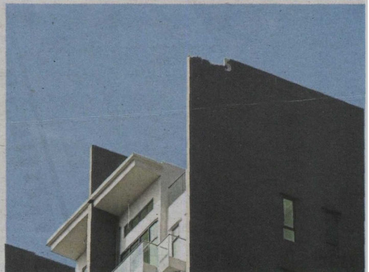
Sometimes, lightning damages corners and pointed features of buildings as seen in this photo.
