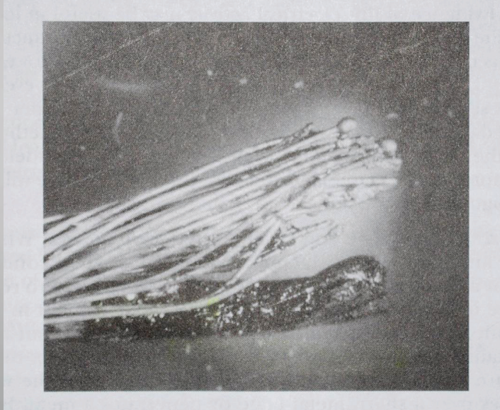
Fig : Stranded Copper Lamp Cord That Was Severed by a Short Circuit
