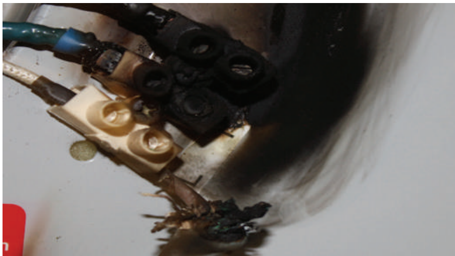
Figure A.2: The burnt condition of connector at the water heater.
