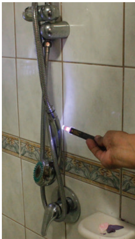
Figure A.3: Metallic water heater hose that was still in an energized condition after the accident.
