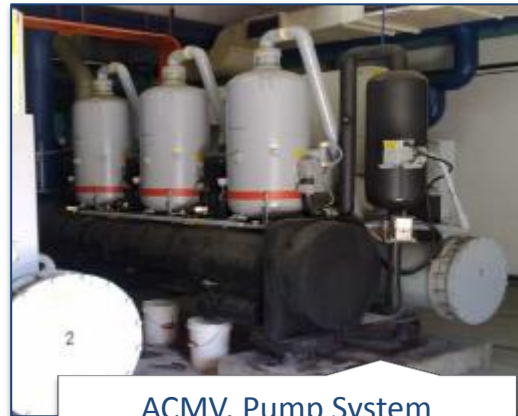
ACMV, Pump System Optimization, Lighting System, Energy Monitoring System
