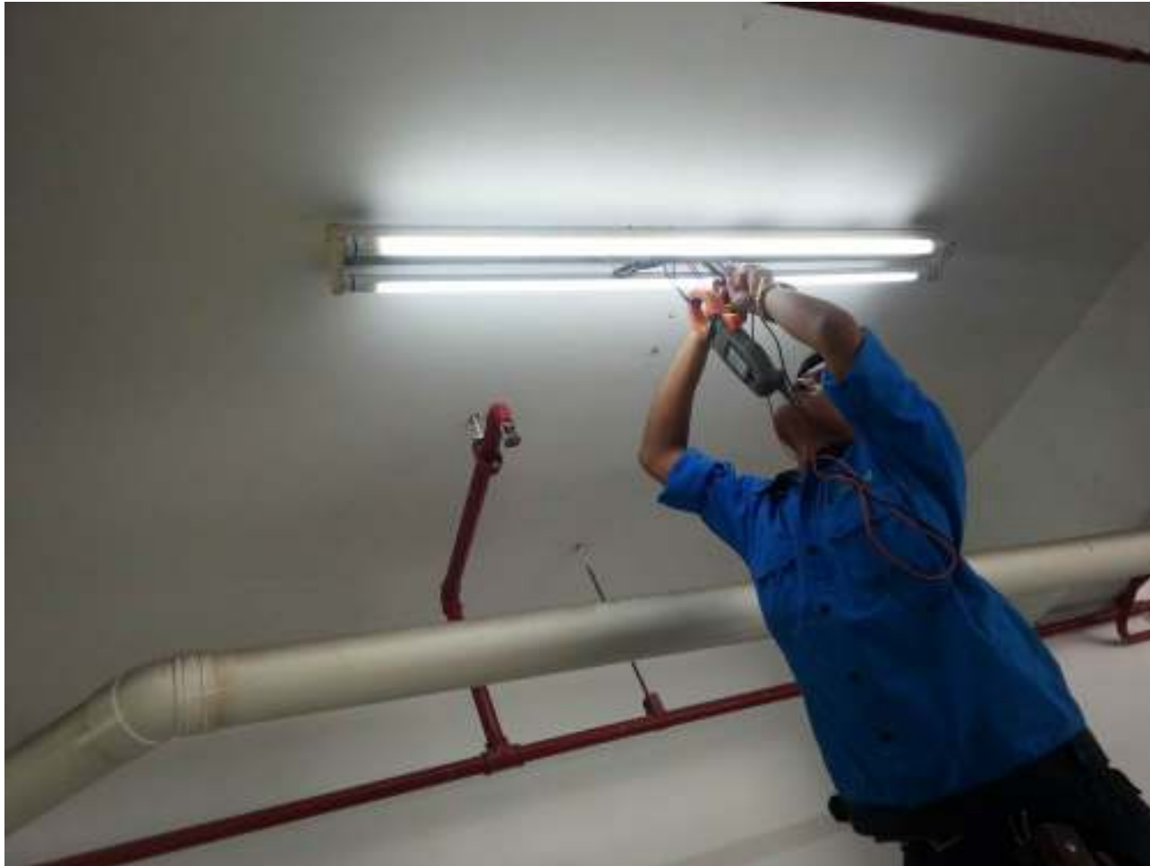
Measurement of energy consumption on the lighting
