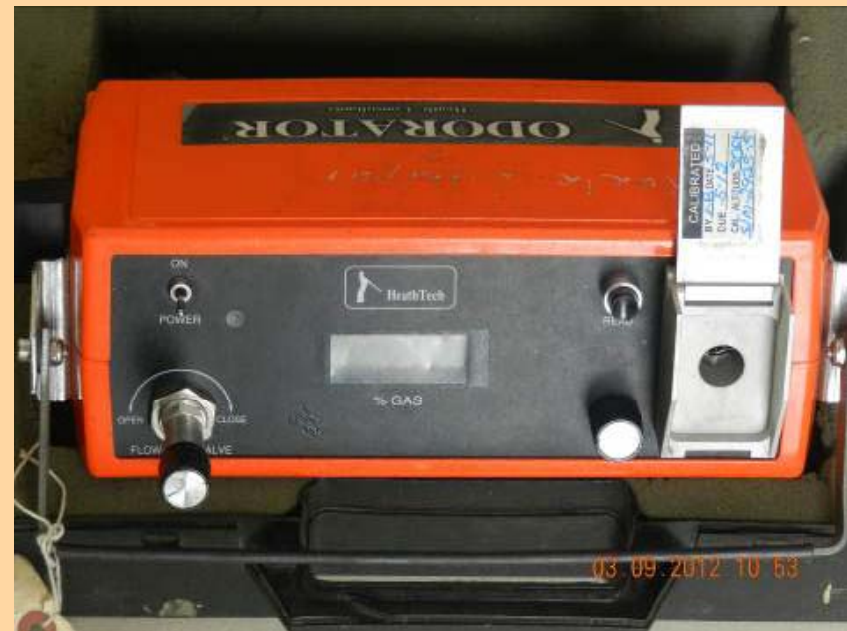
Figure 4.7: Odorator for Gas Detection Control and Monitoring Console
