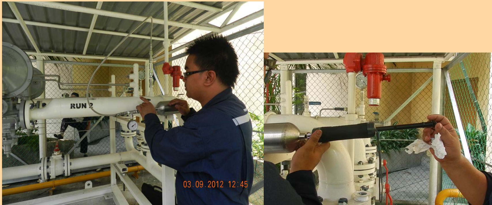
Figure 4.5: Pump Intake Stroke for Gas Sampling Measurement
