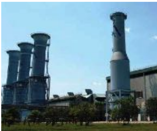
Putrajaya Power Station is a gas turbine plant that had an original installed capacity of 625MW; currently only 270 MW is still operational.
