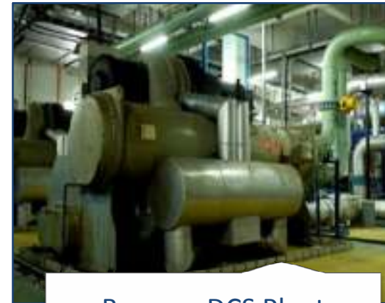
Bangsar DCS Plant (Bangsar Energy System)
