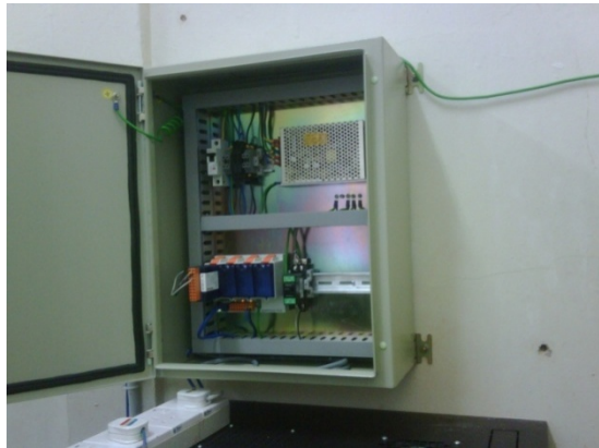
Power Monitoring System (2 system)
